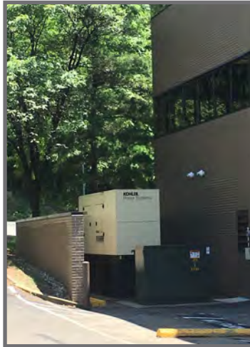
Back-Up Generator (200 KW, 301 AMP Diesel)
